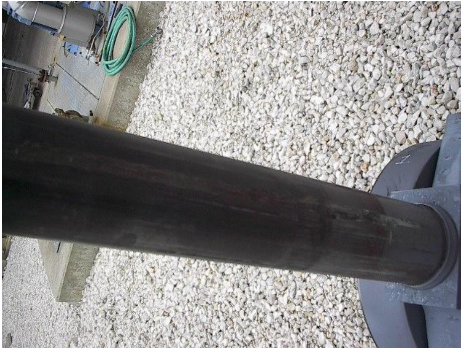
As found stem showing damage to packing area
